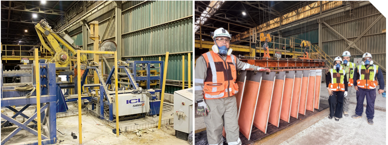
Figure 9 | (Left) The ICL robotic harvesting arm at Sierra Atacama; (right) cathode harvested from the new stainless-steel plates, August 2026.
