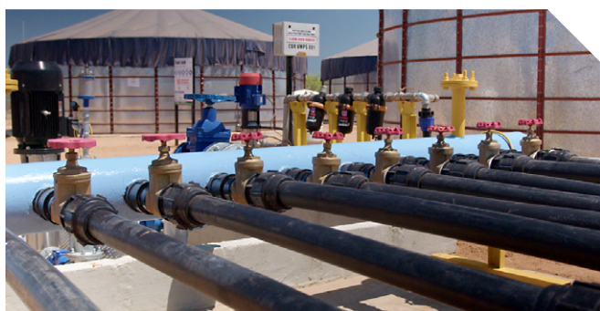
Figure 20 | Ngami ISCR well field – injection and abstraction pump manifold, tank farm and SCADA-controlled infrastructure, delivered with contractor Mitchell Group.
