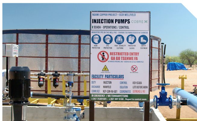
Figure 21 | ISCR well-field injection pumps under SCADA operation and control, Ngami.
