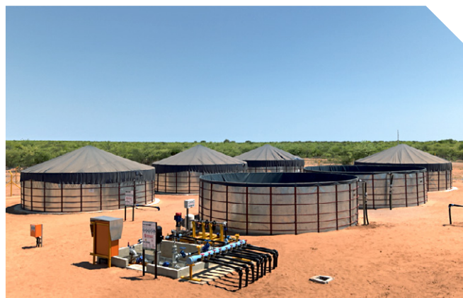
Figure 23 | Tank farm and injection control hub, Ngami.
