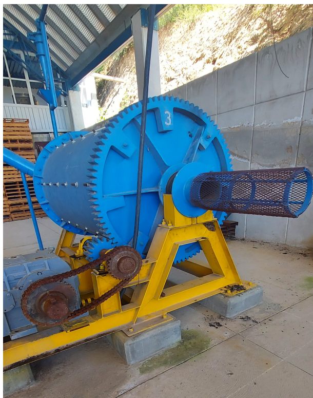
Figure 8 - Tecamatlán Plant – Ball Mill #1
