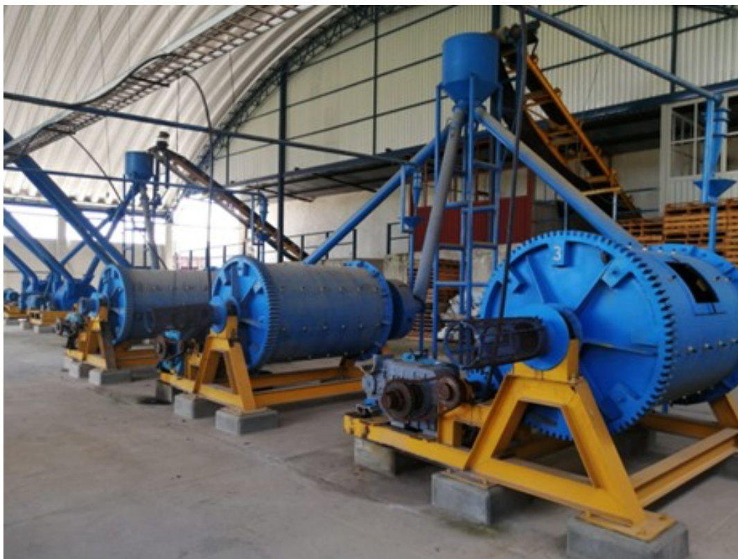
Figure 2 - Tecamatlán Plant – Grinding Circuit, Ball Mills
