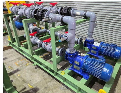
Regen Liquor Transfer Pumps Skid
