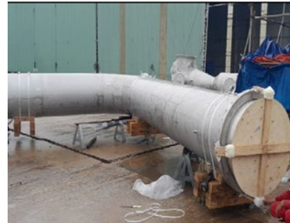
Main Ducting to Venturi Scrubber
