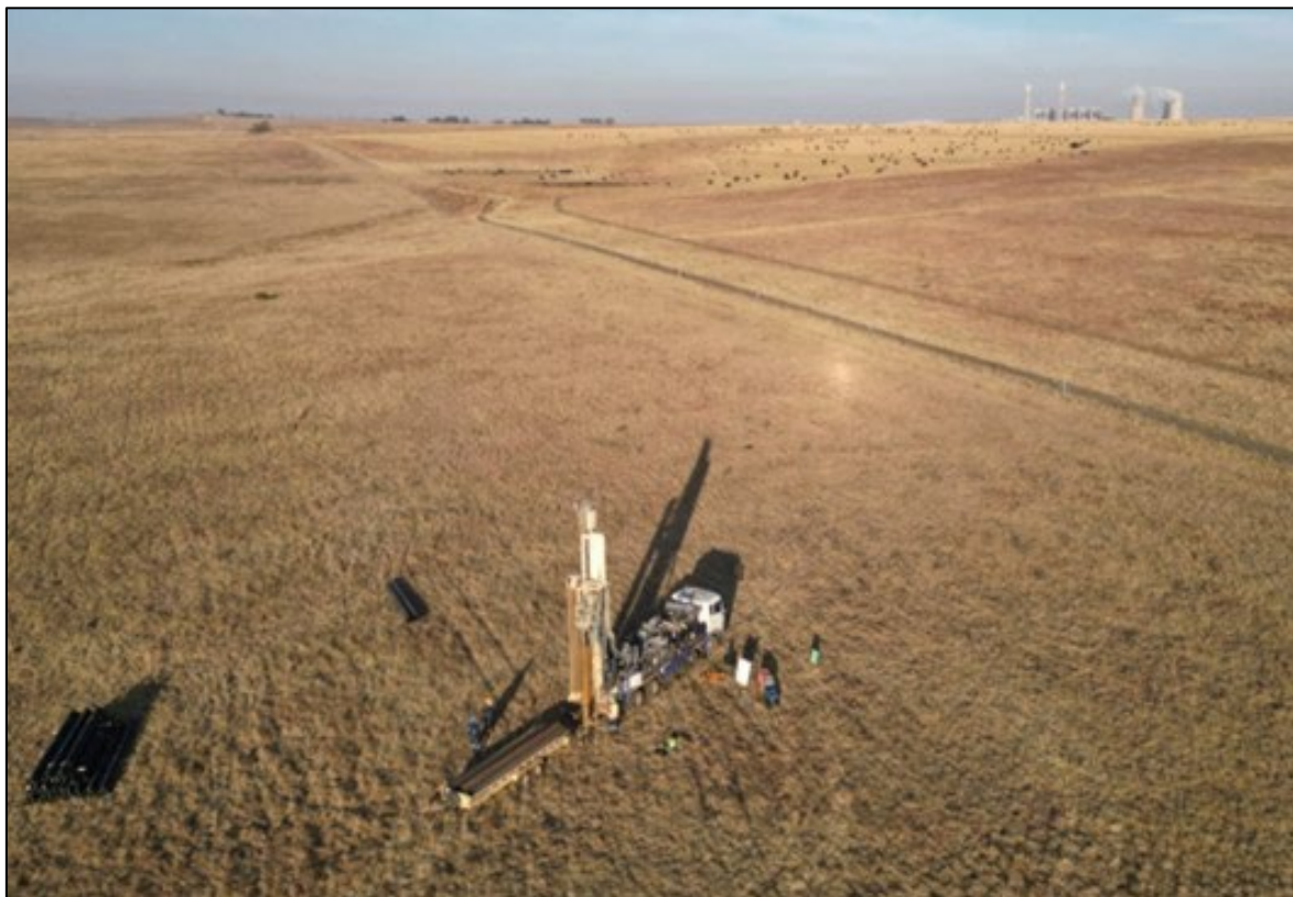
Figure 1: Drilling rig and consumables arriving on site with Majuba power station in the background
