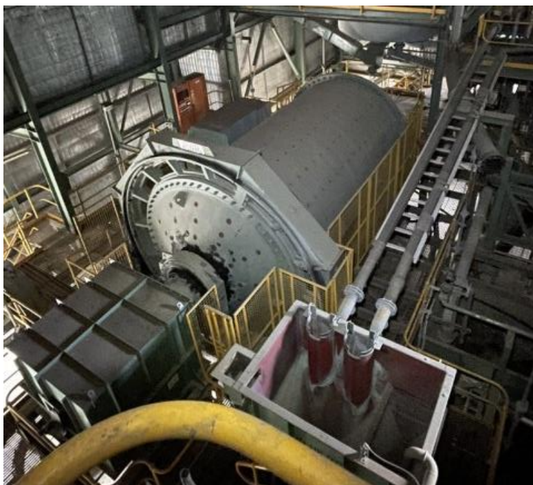
Figure 7: 750kW Outokumpu ball mill (April 2024) prior to being transported to the Murchison.
