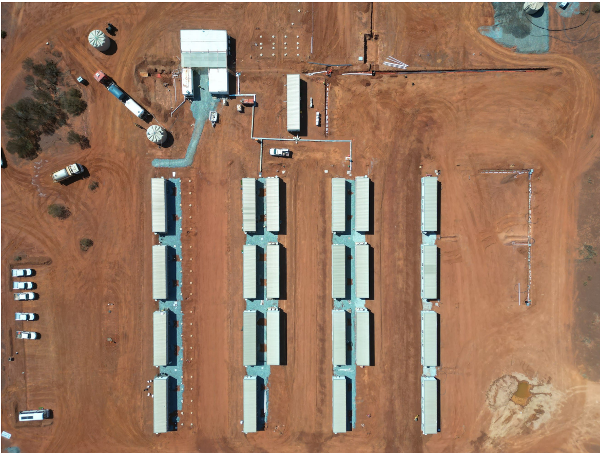
Figure 5: Drone image of the accommodation village. Construction progressing well with 88 rooms installed of a total of 136 rooms.
