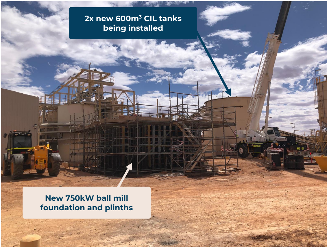
Figure 2: New ball mill foundation and plinths for larger 750kW ball mill, December 2024.
