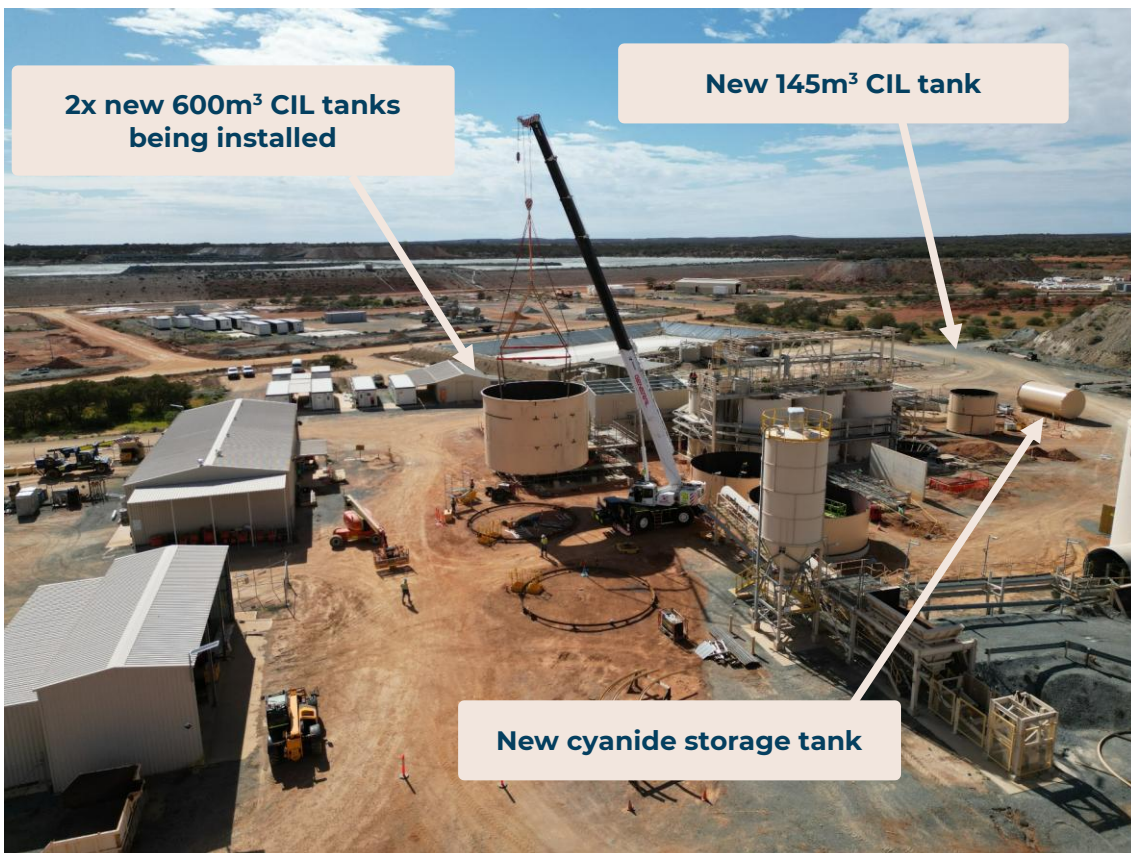
Figure 3: The 2x new 600m³ tanks being installed for the expanded CIL circuit, December 2024.
