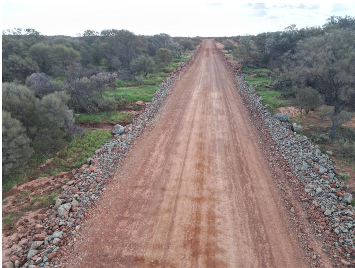
Figure 9: Example of upgraded section of haul road between the processing plant and the open pit mining area with rock armouring on shoulders to ensure long term resilience during wet weather events, January 2025.
