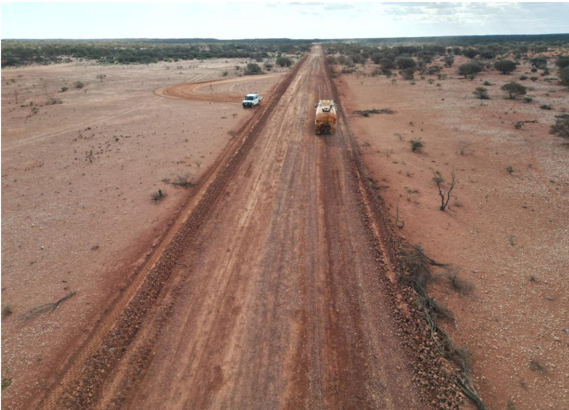
Figure 8: New 20km haul road between the processing plant and the open pit mining area in anticipation of open pit mining fleet mobilising, January 2025.
