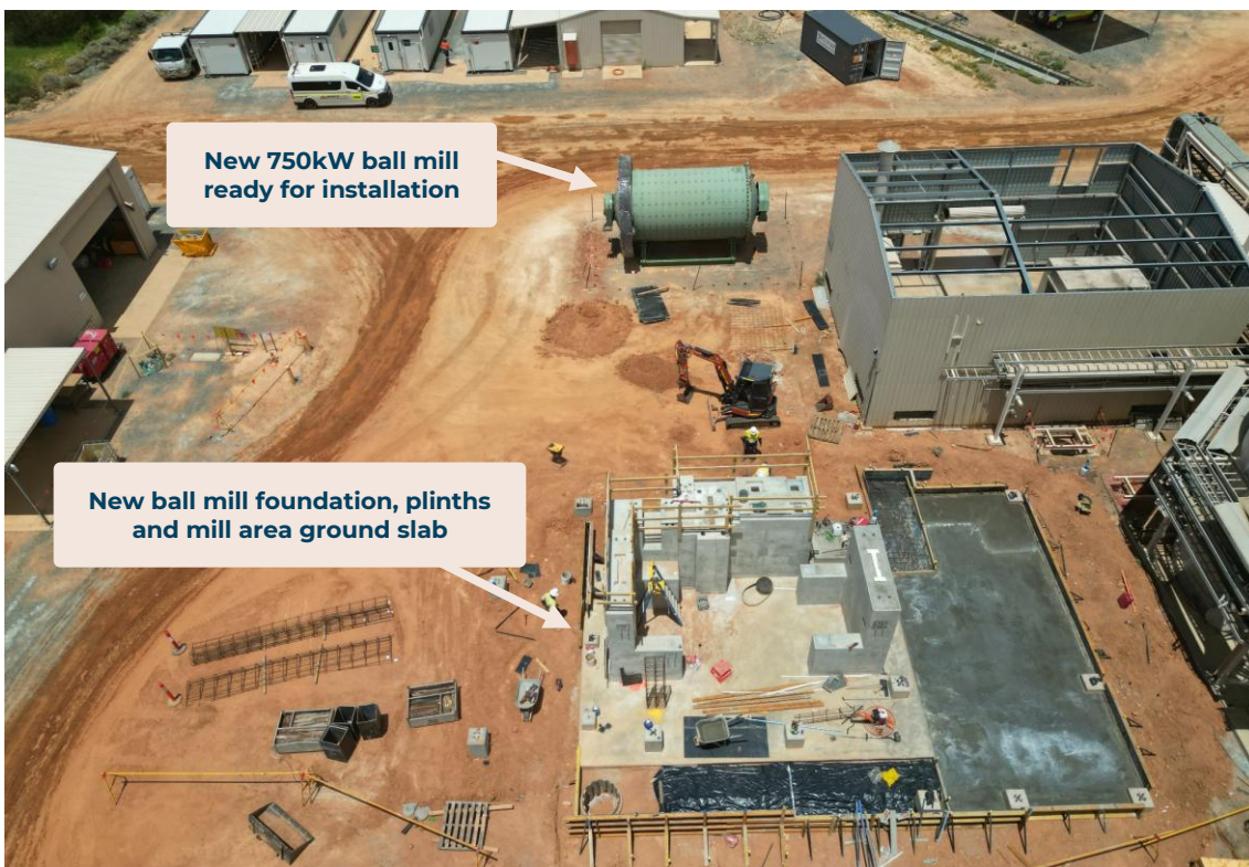
Figure 2: Formwork and scaffolding stripped from new ball mill plinths and mill area ground slab poured, January 2025.
