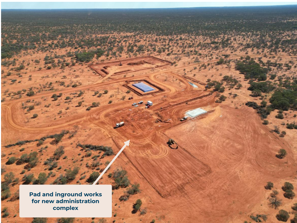
Figure 6: Civil works underway for the new Turnberry administration complex to accommodate open pit and underground operations, January 2025.
