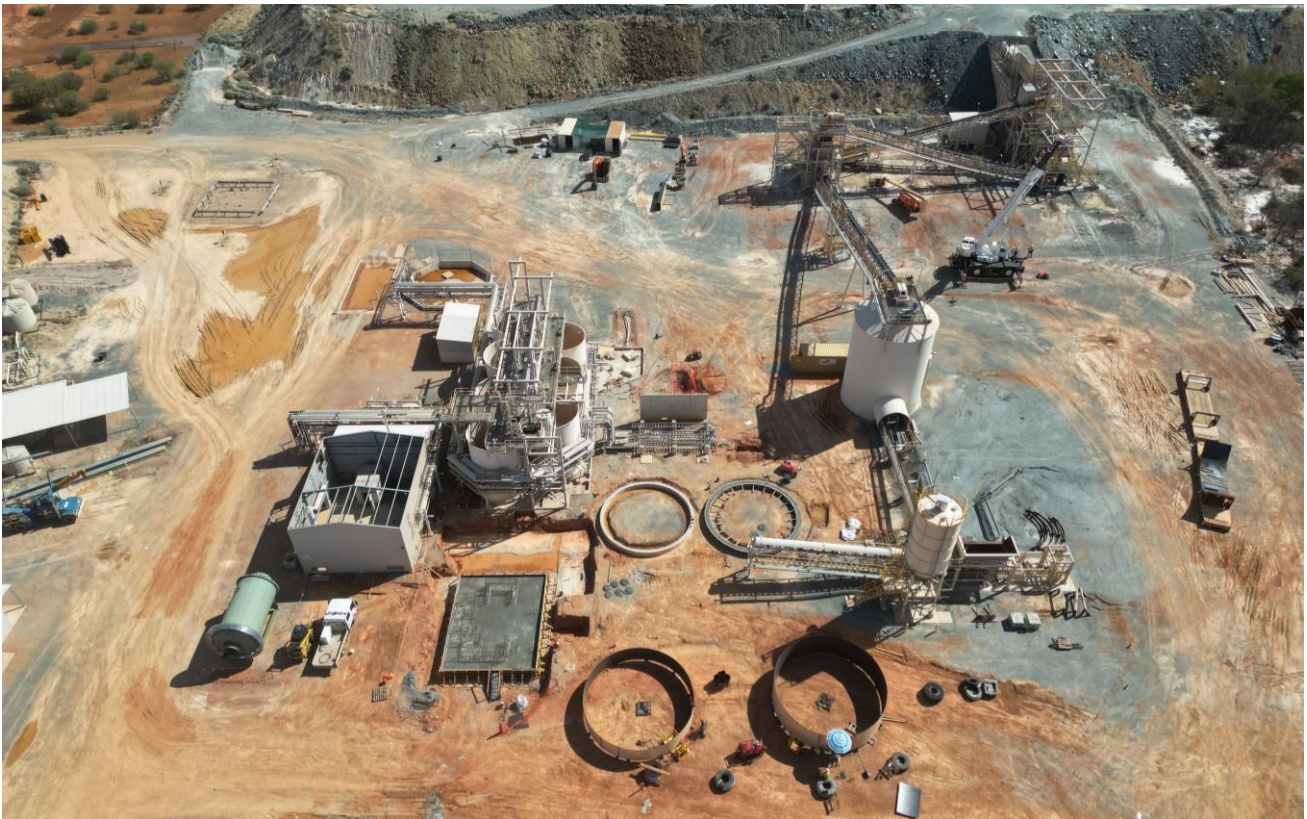
Figure 41 – View of the new leach and adsorption tank foundations and tank skins being fabricated (November 2024).
