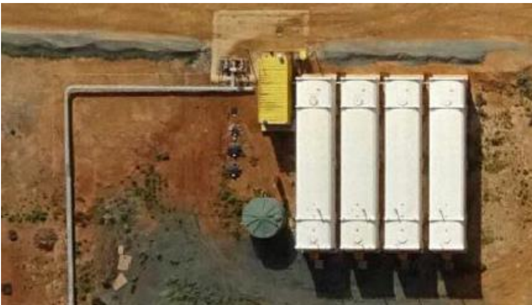
Figure 53 – Andy Well Fuel storage setup (tanks need to be reinstated).
