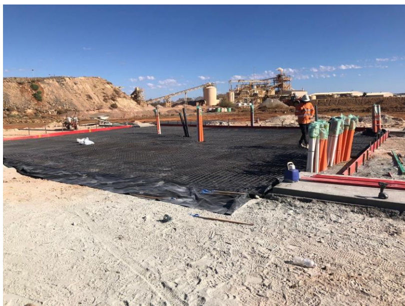
Figure 4: Ore sorter pad with electrical supply conduit.
