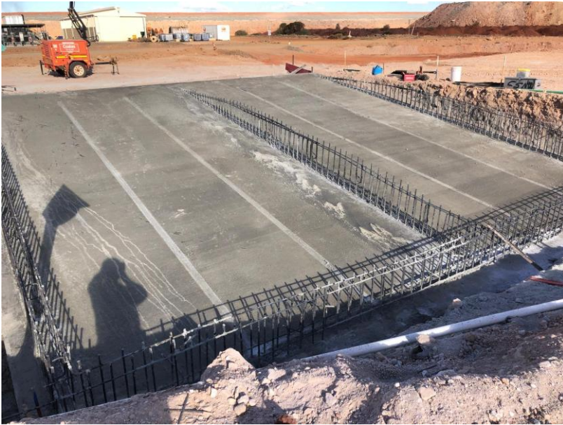
Figure 6: Wash plant sumps.
