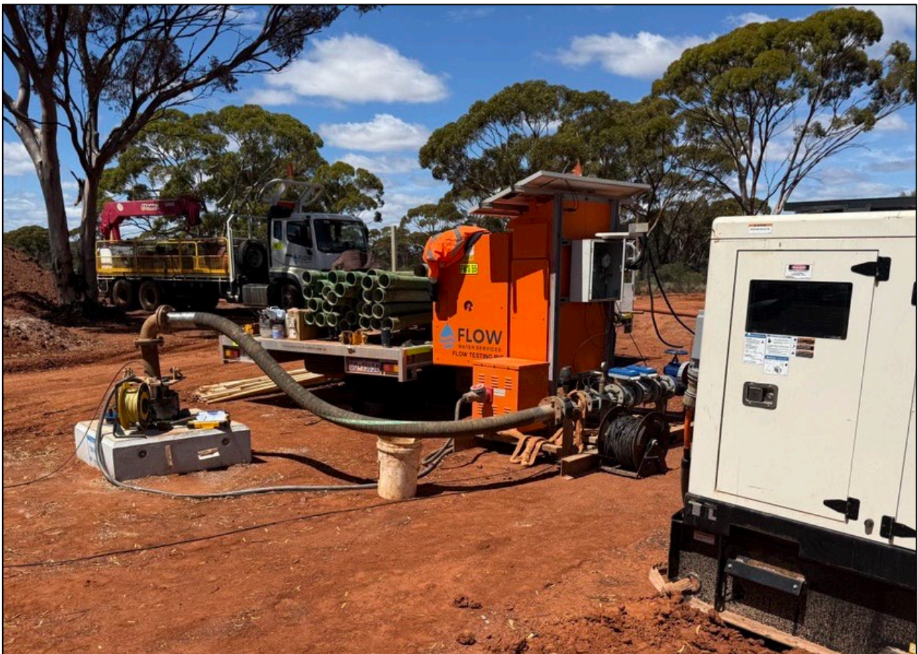
Figure 6: Southern Borefield – water bore pump testing
