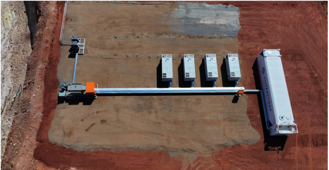
Figure 5 – Main and Pollard temporary power station
