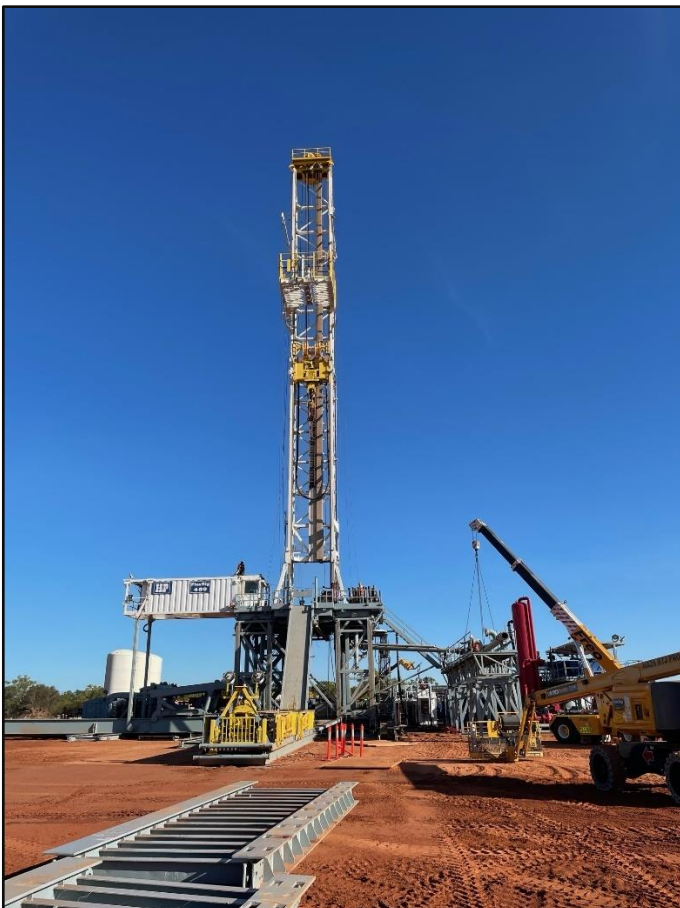
Figure 3: H&P's super-spec FlexRig® Flex 3 rig on location at the SS2 well pad
