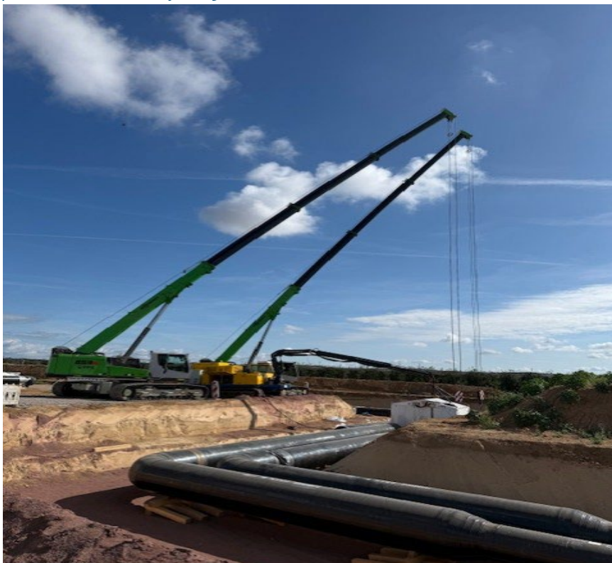
Figure 8: ICPP elbow section in the double walled and steel cased pipe transporting lithium brine and industrial water between well sites and processing facilities.
