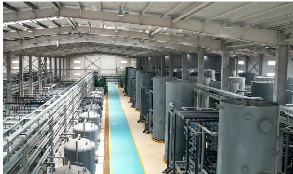
CHINA - EVEBATTERY A-DLE PLANT
