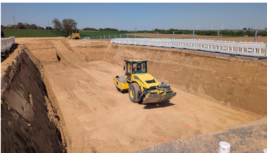
Figure 3: Construction works at the fourth production site ahead of mobilisation of the V10 rig in H2 2026.
