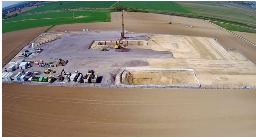
Production well site near Landau
